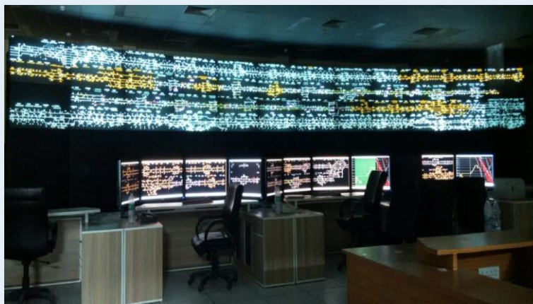
Figure 3: Operations control centre Tundla, North Central Railway
